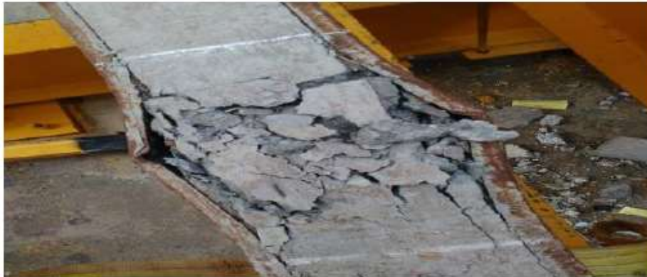
Plate 1. Buckling of steel in compression zone
