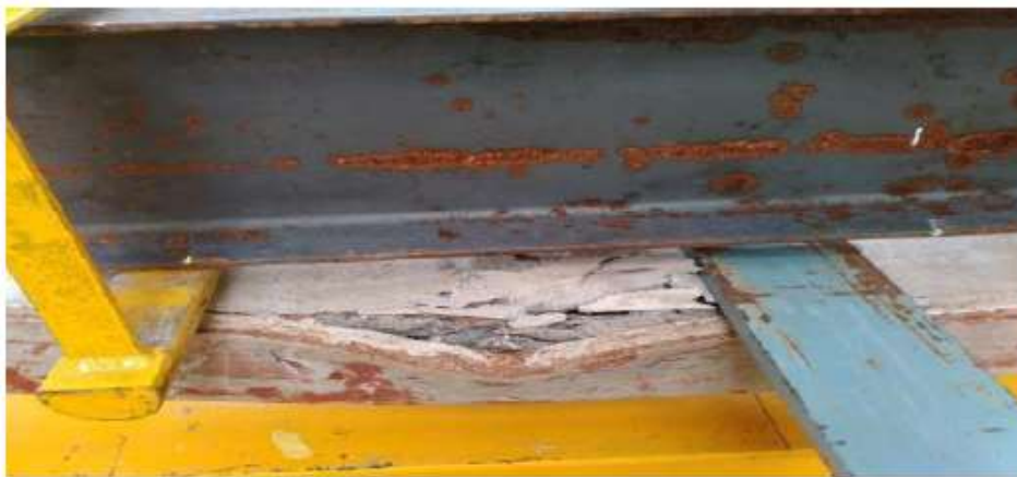
Plate 2. Separation of concrete and steel
